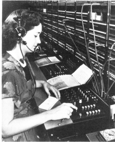
Fig. 3-39. Switchboard position with keyset.
