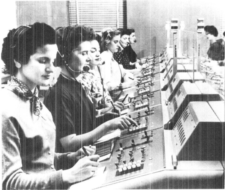
Fig. 10-3. New York Telephone Company trial in Poughkeepsie, New York of positions allowing operators to service many types of customer-dialed calls.
