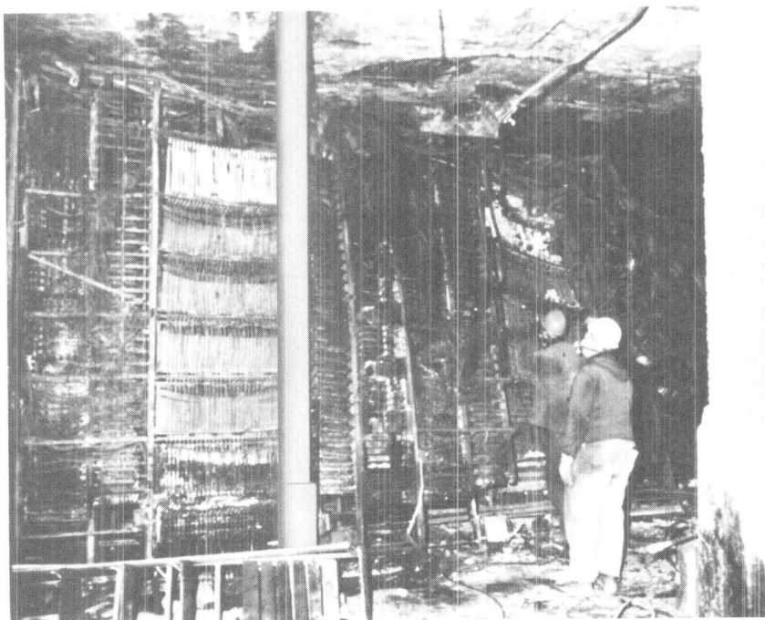
Fig. 11-53. Panel switching equipment damaged in the disastrous February 1975 fire in New York City. Large Bell System resources were employed to restore service quickly.
