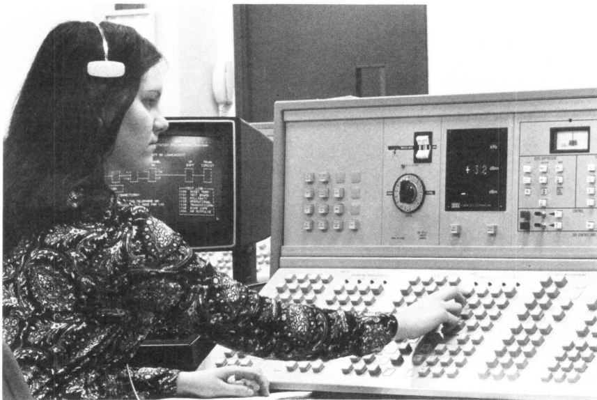
Fig. 12-7. Barbara Reed, Long Lines, at a 51A test position of the circuit maintenance system 1A, which gives craftspeople access to No. 4 ESS data bases and circuits for trunk maintenance.
