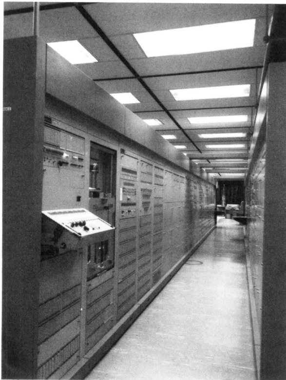
Fig. 9-47. Row of UNICOM switching equipment which employed forced air cooling, an example of special design to meet military requirements.
