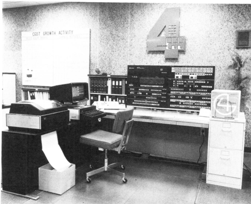
Fig. 12-9. Maintenance operations center at the Chicago 7 No. 4 ESS office. The master control center is also located here.
