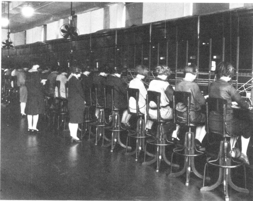
Fig. 3-23. No. 3 toll switchboard, high keyshelf type. Over 50,000 positions of the No. 3 were produced.
