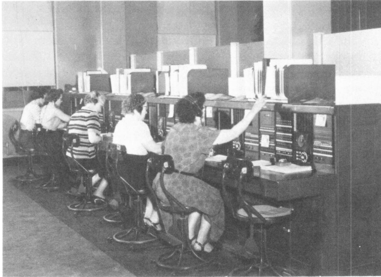
Fig. 11-18. New York City installation of No. 12 service observing desks, developed in 1949 to centralize this function for various central office systems and switchboards.
