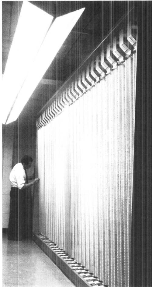
Fig. 11-38. Main distributing frame for No. 1 ESS, requiring one half or less of the space required for earlier MDFs.
